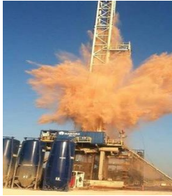
Pressurized lines being improperly connected or being hammered on while under pressure cause 'production fluid spills' Source: MEF n.d.
