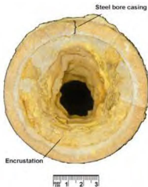
Figure 2 Example of encrustation within a bore (© Copyright, DSE 2004).
