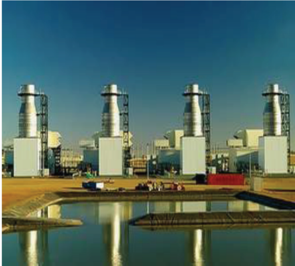
Gas-fired electricity generator
