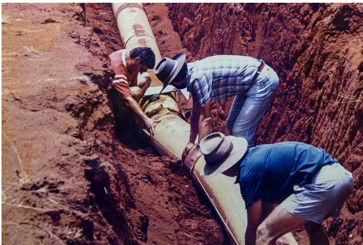
A gas pipeline is repaired after the 1988 Tennant Creek earthquake. Photo: Geoscience Australia in
