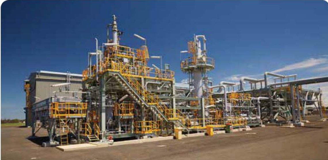
Condabri Central gas processing facility
