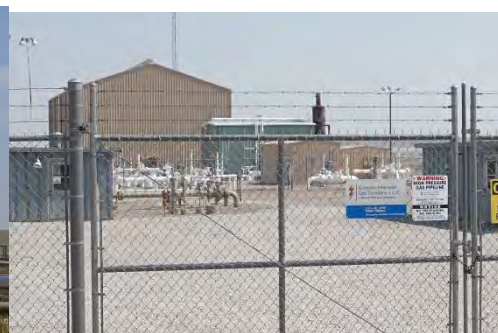
Colorado Interstate Gas Company Treating Facility
