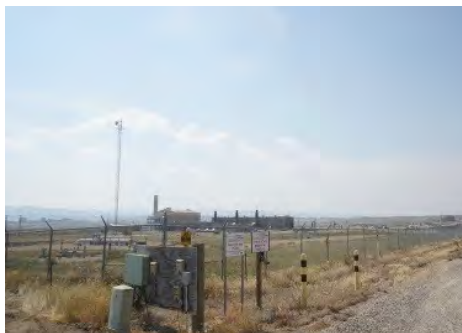
Fort Union Gas Gathering Plant
