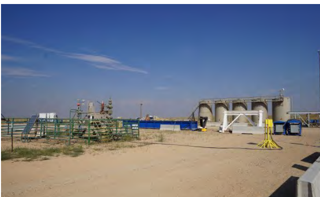
Single well (left) - condensate tanks on the right
