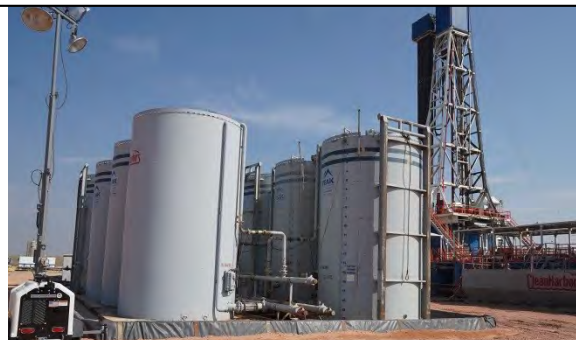
Drilling fluids stored in tanks sitting on plastic liner bunker
