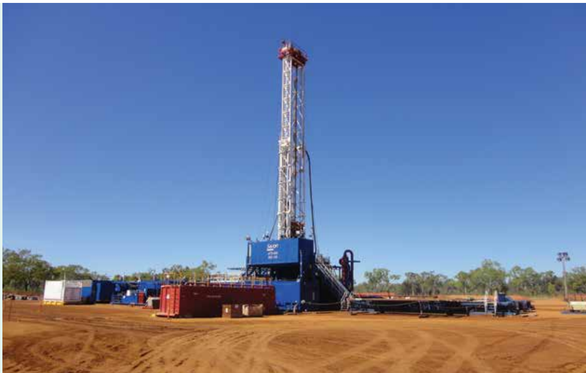
Drilling Rig at Kalala S-1 exploration well. Identical drilling rig also used at Amungee and Beetaloo well sites. Source: Origin.
