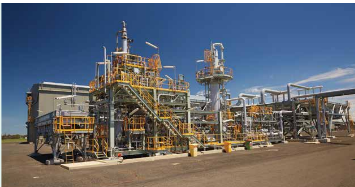
Condabri Central Gas Processing Facility. Source: Origin.
