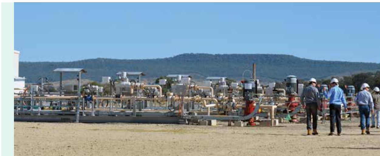
Multi-well pad infrastructure (CSG), Roma Queensland, as visited by the Panel, July 2017.
