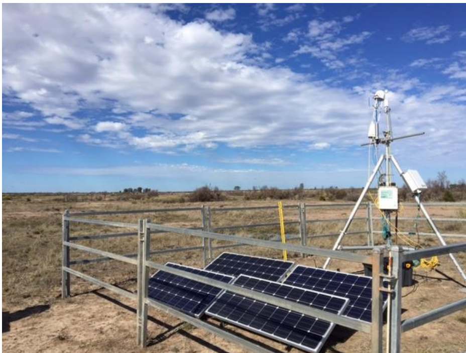
Figure 11.2 - A Licor Eddy Covariance methane measurement system installed adjacent to an Origin CSG well by Macquarie University. These stations are solar powered and were utilised to estimate the entire life cycle of fugitive emissions from drilling through to production. https://researchdata.andcs.org.au/linkage-projects-grant-id-lp140100460/618640
