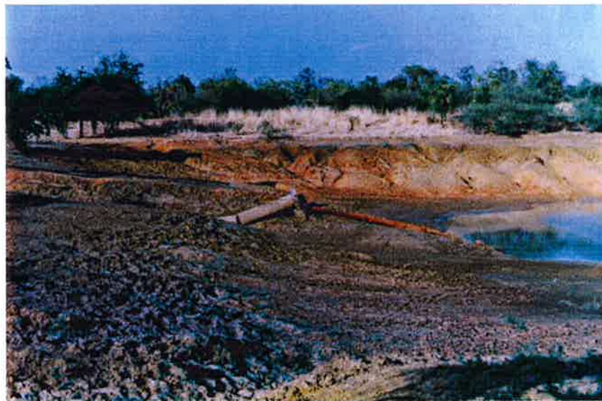
Plate 12 Four Mile Dam, Auvergne, the embankment has been damaged around the inlet pipe by flood waters.
