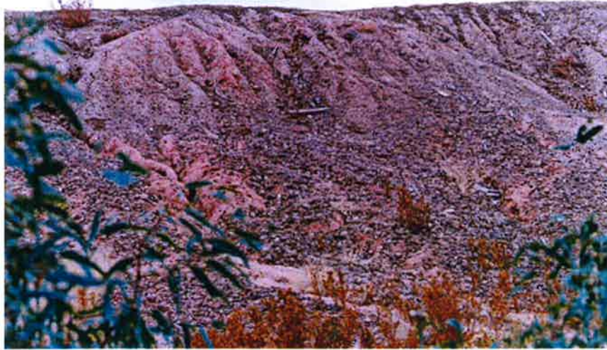
Plate 13 Rill erosion of the embankment of No.2 Dam, Auvergne.
