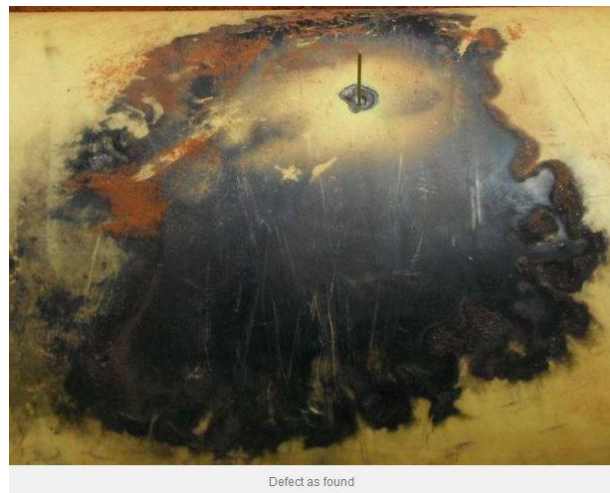
Defect as found
